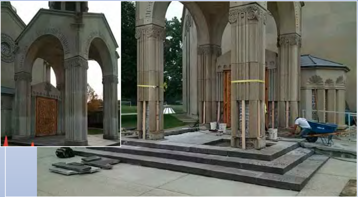
St John's Armenian Church Limestone and Granite Restoration 2016 Submitted by: JMD Building Restoration / Joseph M. Dapkus Jr.
